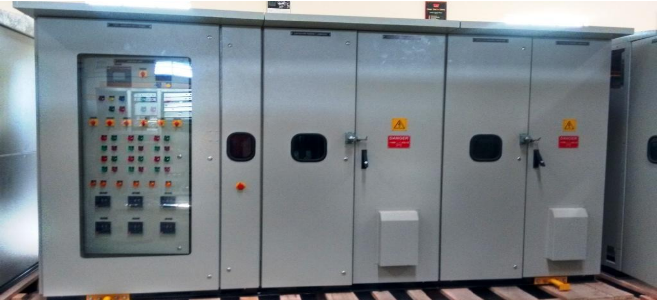
HT CAPACITOR PANELS:
