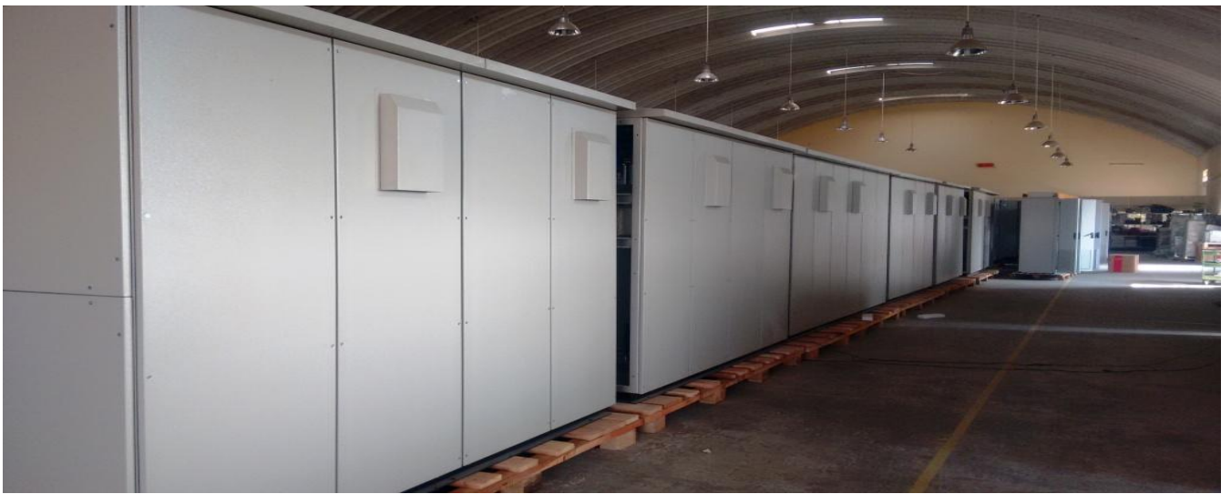
SIKAP CAPACITOR PANELS :
